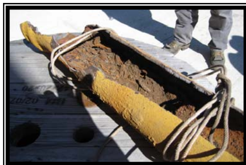
In this photo, decay in a recently replaced wastewater pipe is shown.
