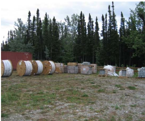
Line material for 138 kV tie to GVEA
