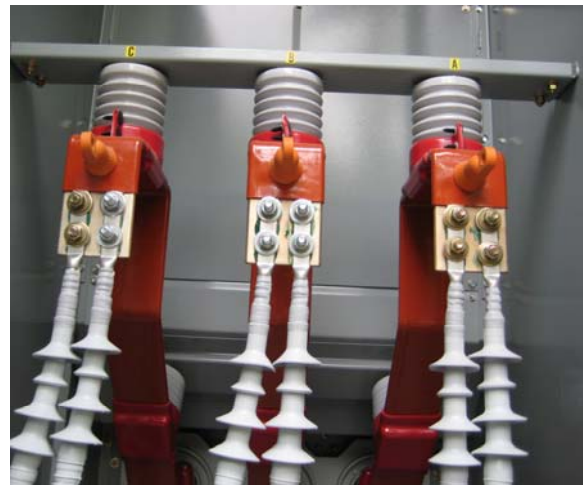
Distribution Feeder Terminations on Substation
