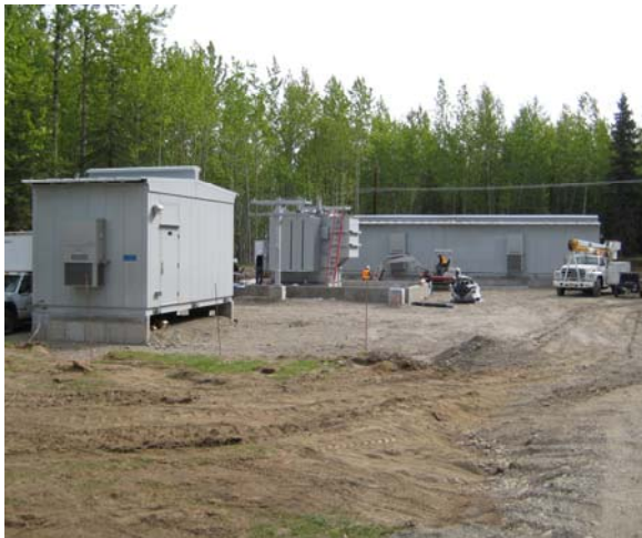
Major Components of FRA Substation
