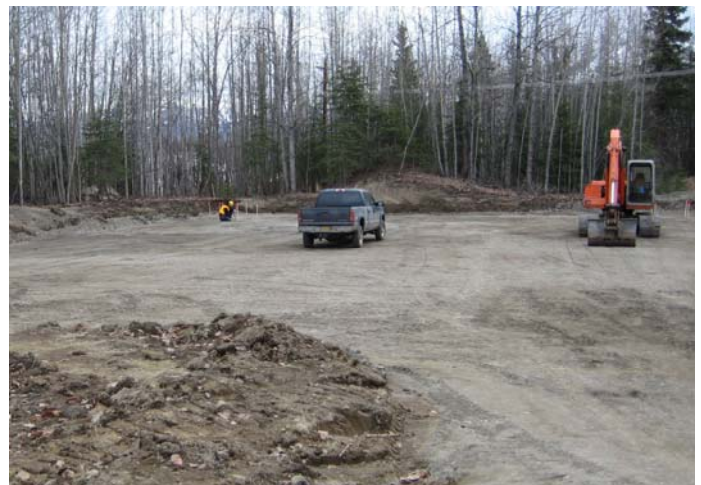
Fort Richardson Substation crew members survey the placement of concrete footings. The substation is scheduled to be moved to this location within the next few days.
