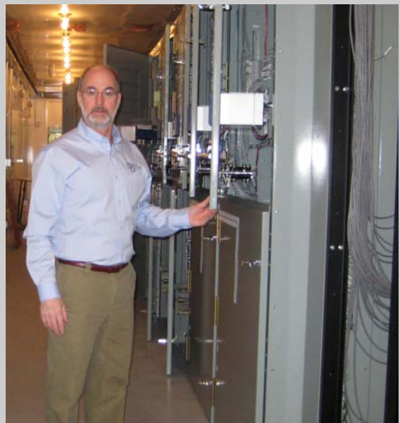
Shayne Coiley, Doyon Utilities Project Manager, poses with the new FRA switchgear in Corona California. For more information regarding this equipment, read the article accompanying this picture.
